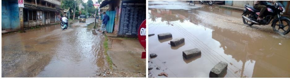
Condition of road after rain in Vakkom Market Jn
